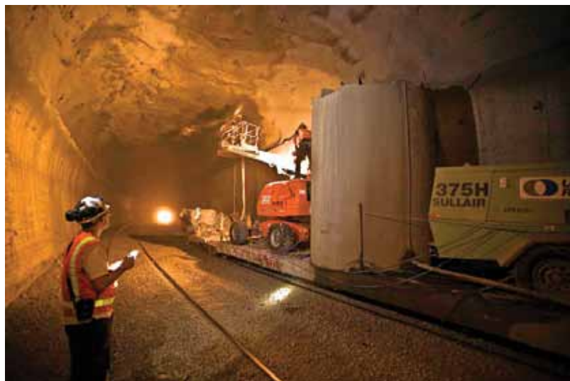
Along the Heartland Corridor, Norfolk Southern has employed a number of methods to increase the clearance, including raising the roof and lowering the track. To expand the tunnels, workers must also transform the passageways' corners from rounded to squared, which allows the taller trains to pass
