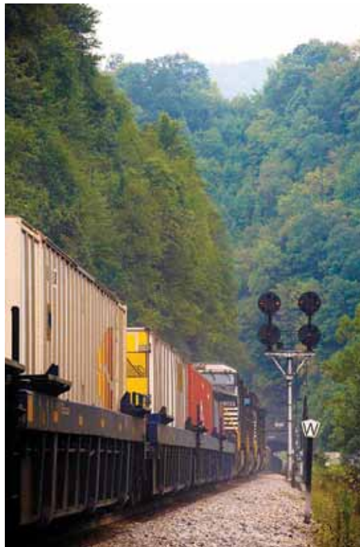
As part of a 3-year project, Norfolk Southern is expanding 27 tunnels along the Heartland Corridor by adding up to 2 ft (0.6 m) of headroom, which will allow larger trains to use the route and cut roughly 200 mi (321 km) off their trip
