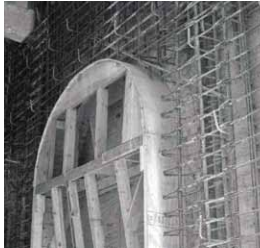
Wooden window form and reinforcement prior to receiving 12 in. (304.8 mm) of concrete
