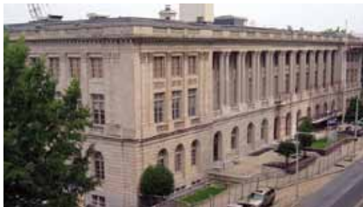
East façade of the University of Memphis' Cecil C. Humphreys School of Law during the renovation project
