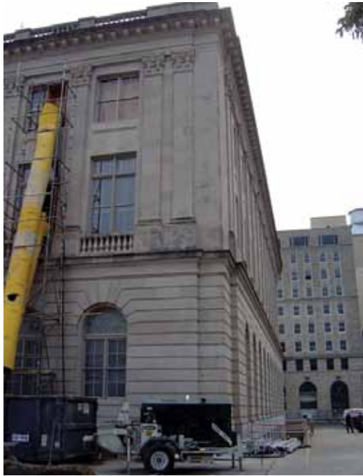
Concrete pump at the southwest corner of the Cecil C. Humphreys School of Law
