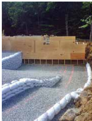
Stone-filled bags used to create floor profiles of pool and catch basin
