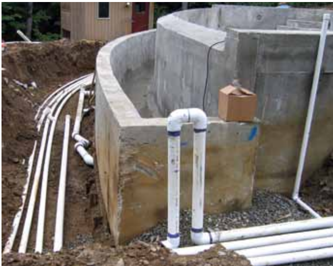
Large diameter plumbing to reduce water velocity and increase efficiency
