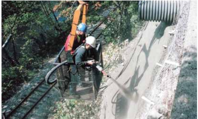
In this slope stabilization in Westernport, MD, the shotcrete conforms to the irregular rock surface
