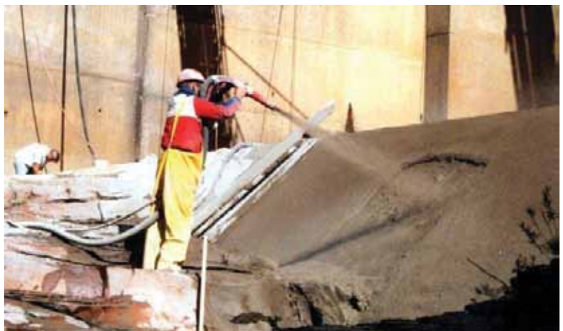
Using the dry process, the nozzleman guns the lower section of the Two Lick Dam in Indiana, PA, with shotcrete. The material is efficiently placed without having to form the repair areas
