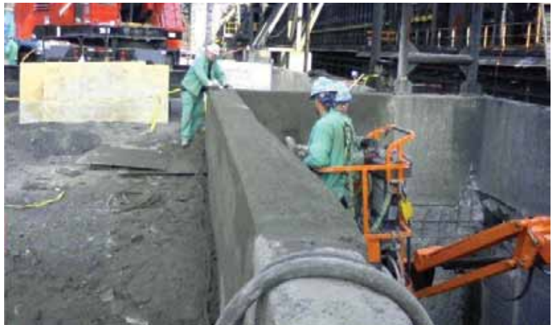
Using dry-process shotcrete, the walls of the sump are easily repaired without forming. The newly placed shotcrete is cut down to grade with the edge of a trowel
