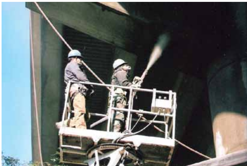
Overhead shotcrete repair on a bridge pier near Pittsburgh, PA, provides a cost-effective repair to existing structures that can prolong the life of the structure
