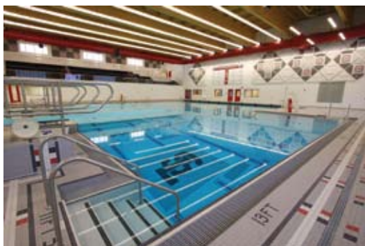
The all ceramic tile competition pool: eight lanes by six lanes, 4 to 13 ft (1.2 to 4 m) deep. The pool walls, steps, and gutter are all shotcrete
