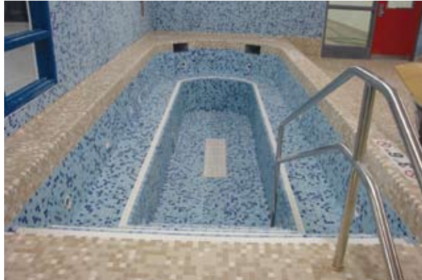
The shotcrete spa with the tiling just finished and almost ready to fill
