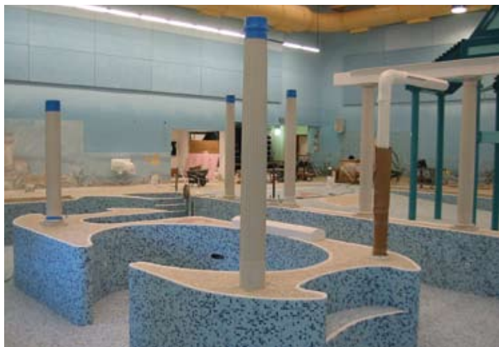
The lazy river island, twirl pool, bubble couch, underwater bench seating, and divider wall between the beach entry and the lazy river illustrate the complexity of the shotcrete work for this pool
