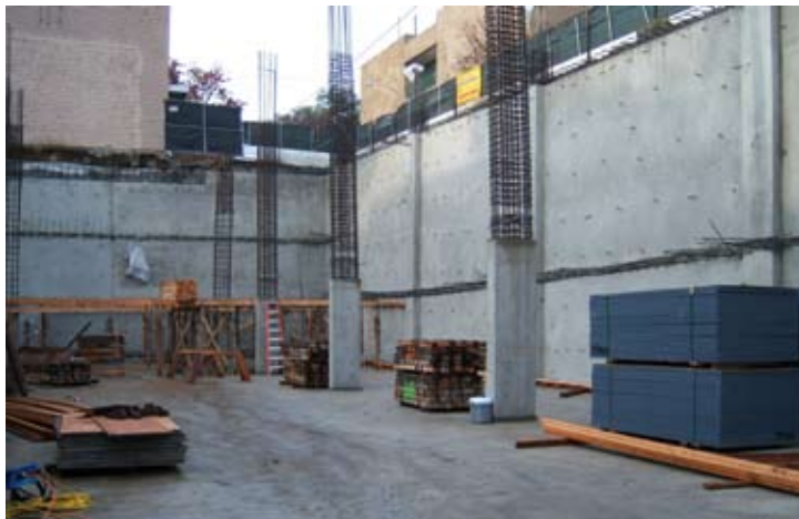
Fig. 4: The shotcrete is placed and finished over the Preprufe® SCS membrane. The completed wall includes grout tubes that are later used to inject the hydrophilic grout for the Preprufe® SCS system (photo courtesy of Johnson Western Gunite Company)
