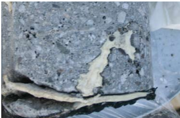
Fig. 3: Core through a shotcrete wall where Preprufe® SCS was used, showing effective grout sealing of voids in shotcrete (photo courtesy of Grace Construction Products)
