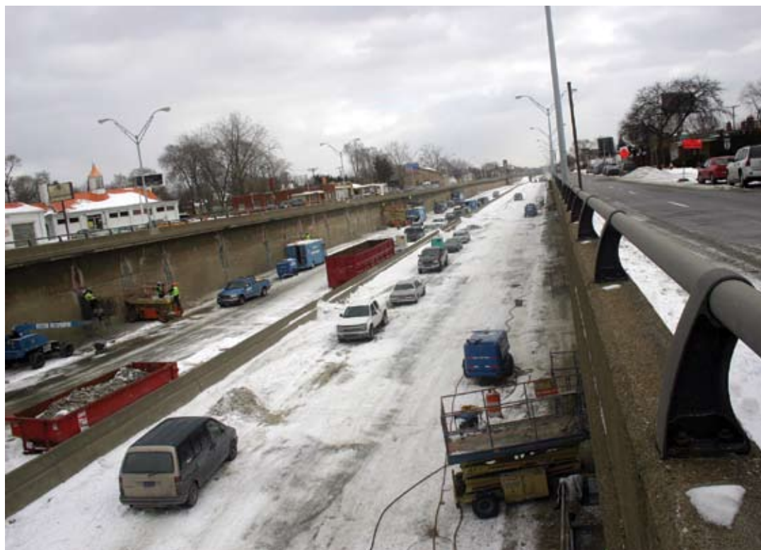
Ram Construction Services had to work under adverse weather conditions in Michigan to complete the project
