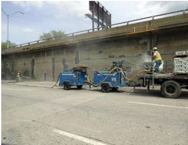
Ram Construction Services shooting during rehabilitation of the MDOT Lodge M-10 Freeway
