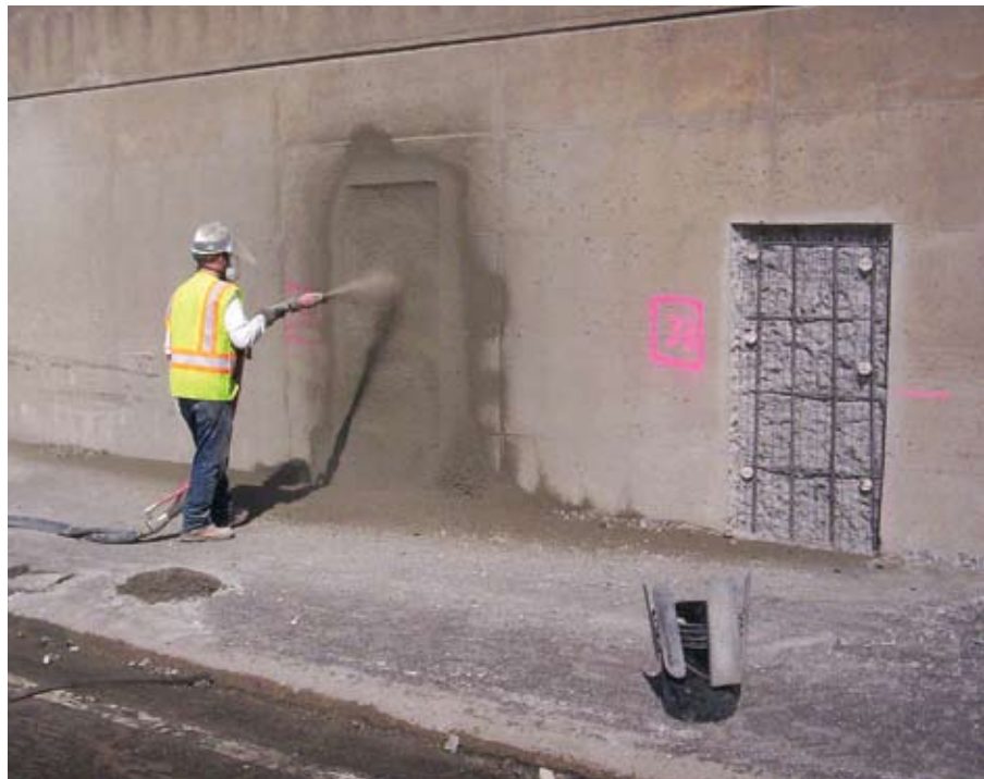
Shooting of prepared area. Note galvanic anodes installed around perimeter of repair area
