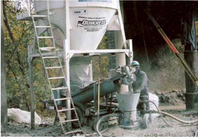
A material hopper with the material being predampened and fed into a rotary gunite machine during shotcrete placement
