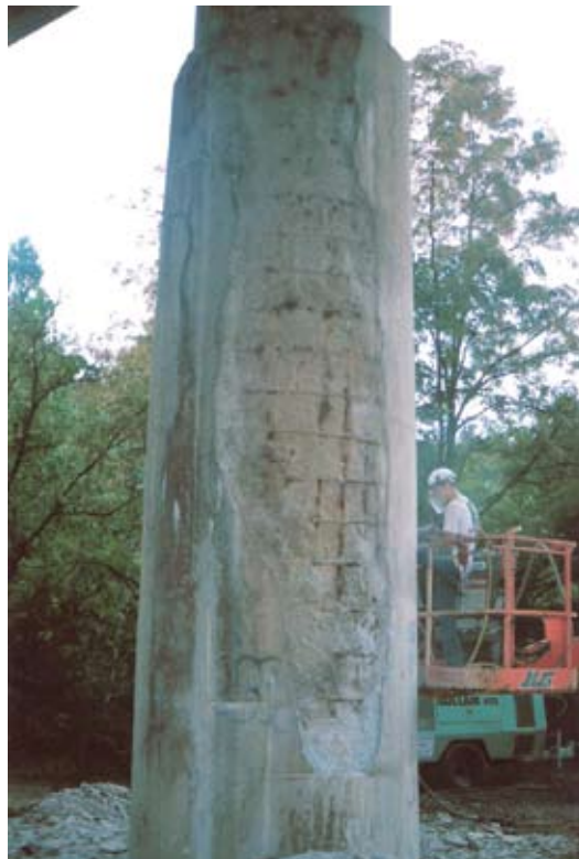
A badly deteriorated bridge pier
