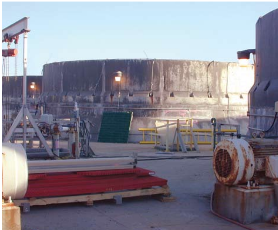
Project No. 2: Fanstack assembly sitting on top of concrete draft cooling towers
