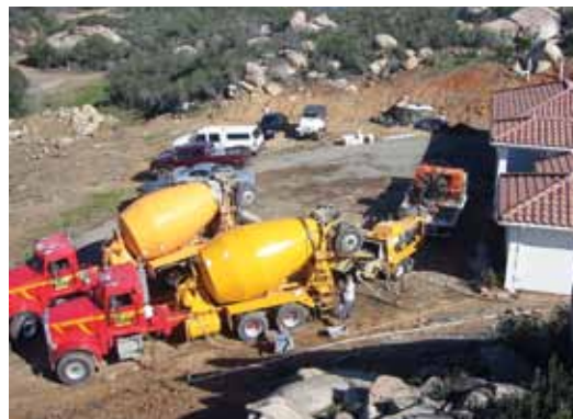
REED C50HP set up and wet-mix shotcrete being pumped for pool construction in Southern California
