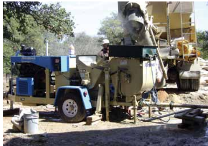
Fig. 3: An Allentown Powercreter 20 is shown with a hydraulic mixer attachment. The attachment is being used as a remixer for concrete supplied by a mobile, volumetric mixer to achieve a consistent mixture for pumping operations. A vibrating screen was installed to reduce the risk of plugging the 1.5 in. (38 mm) hose due to randomly occurring large aggregate particles. The new electronic technology produced a continuous flow of concrete material that allowed the nozzleman to apply a uniform shotcrete layer to the walls with very little line surge
