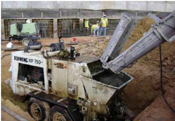
Fig. 5: A Schwing 750 trailer pump that was set up for easy maneuvering in and around the job site
