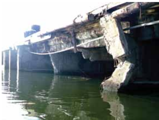
Using one-sided form technology, damaged support members were rehabilitated to their original state after being struck by ships
