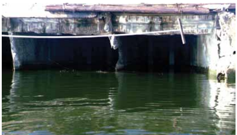
Typical damage to Manchester Terminals prior to shotcrete application
