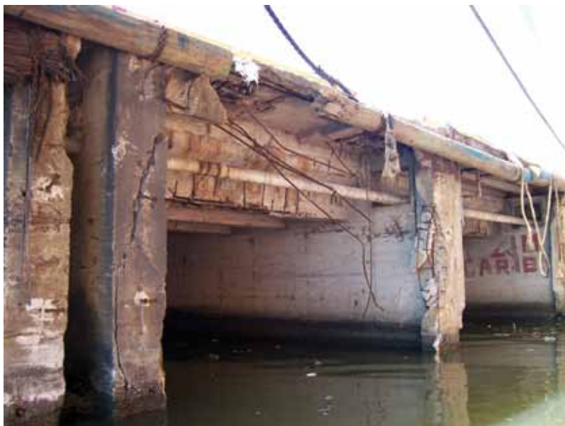
Typical damage due to environmental effects on concrete
