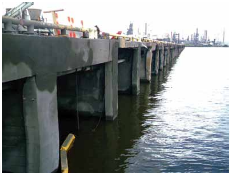
Manchester Terminals dock begins to find new life as shotcrete application progresses
