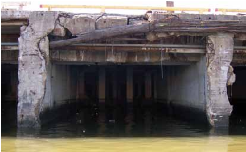
Damage as seen in over 90% of support columns prior to repair
