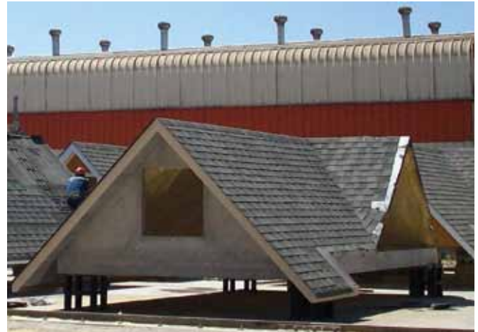
Shingled and insulated Tekcrete roof module ready for painting and window installation
