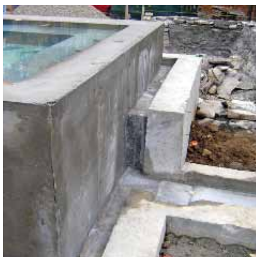
The multi-level runnel system around the spa that will carry overflow water to the pool
