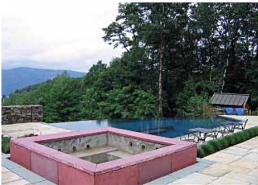
The pool is complete, and the spa is nearing completion as it gets clad with red concrete panels
