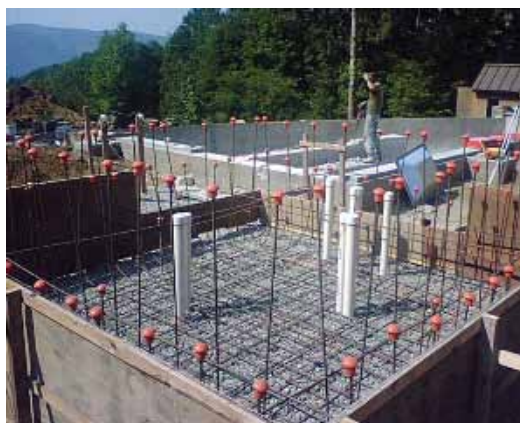
The base of the perimeter edge spa ready for Phase 3 of shotcrete
