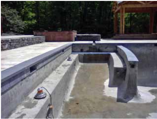
The dividing wall in the pool, along with benches. Coping and tile are being installed
