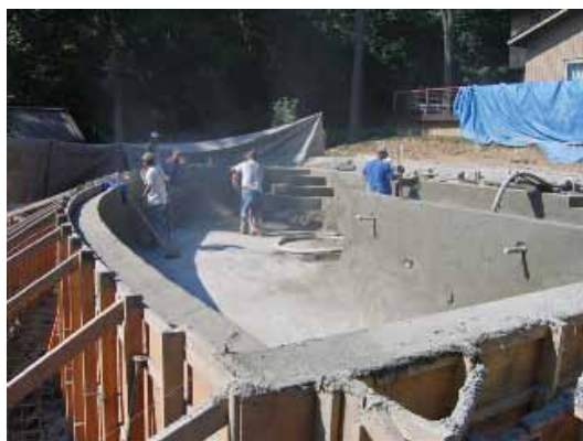
Phase 1 of shotcrete. Note top of freestanding wall is cut to an angle, with dividing wall to the right
