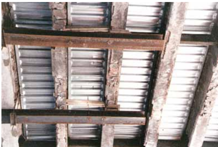
Damaged beams on one of the spans
