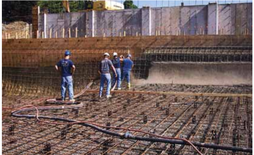
Cove wall and floor intersection on the first day of the project
