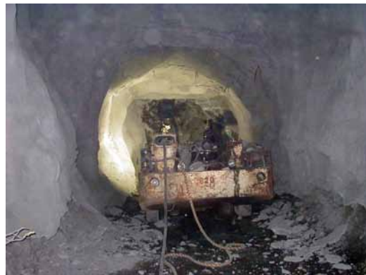
Fig. 15: Shotcreted drift at Creighton Mine (after seismic activity)
