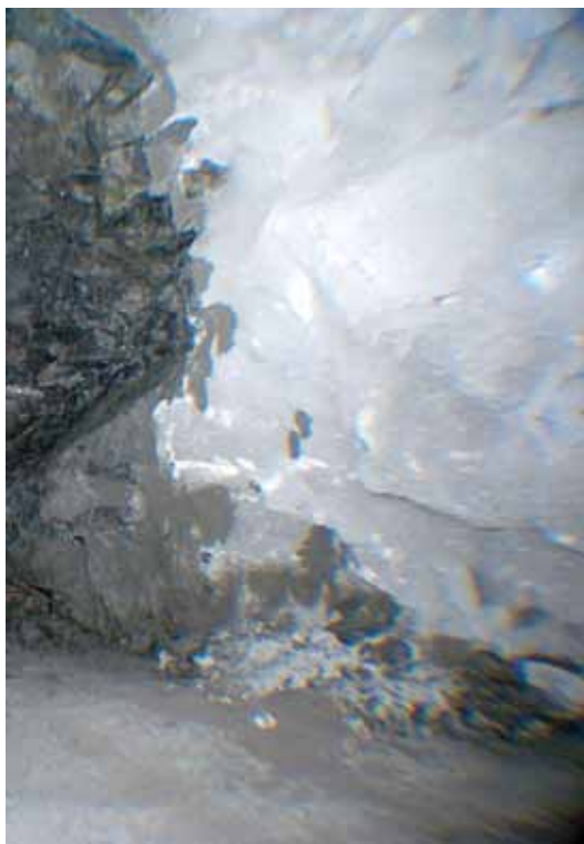
Fig. 1: First shotcrete attempt with cement, sand, and water mixture (mortar-like) showing poor performance with cracking
