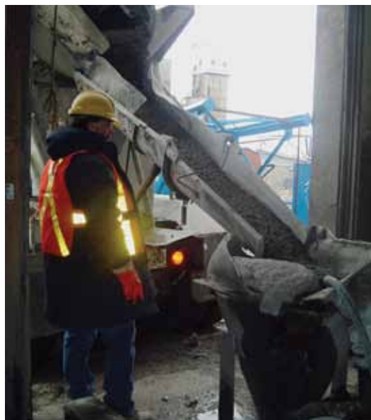
Fig. 16: Wet-mix shotcrete material is delivered from a bore hole on surface and dropped several thousand feet (meters)
