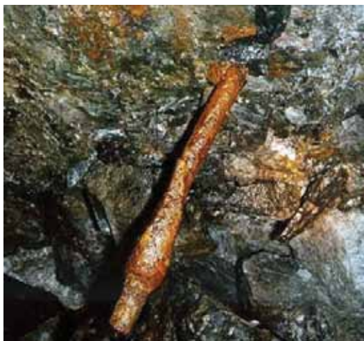
Fig. 5: Corroded screen and bolts
