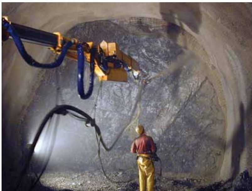
Fig. 4: Shotcrete sprayers increased the comfort level of the nozzelman, improved productivity, and created a safer work environment
