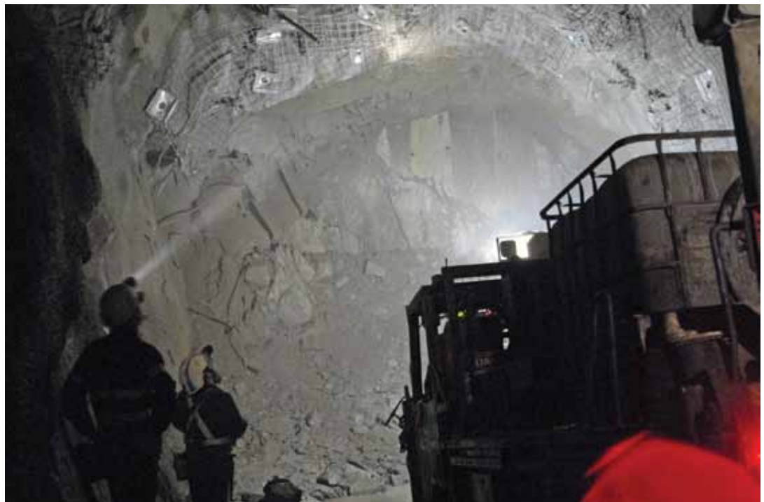
Fig. 7: Very poor ground with high water ingress at LGL Ballarat Goldmine, Victoria, Australia
