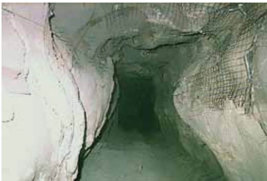
Fig. 5: FRS with mesh over the top in squeezing ground at Perseverance Mine
