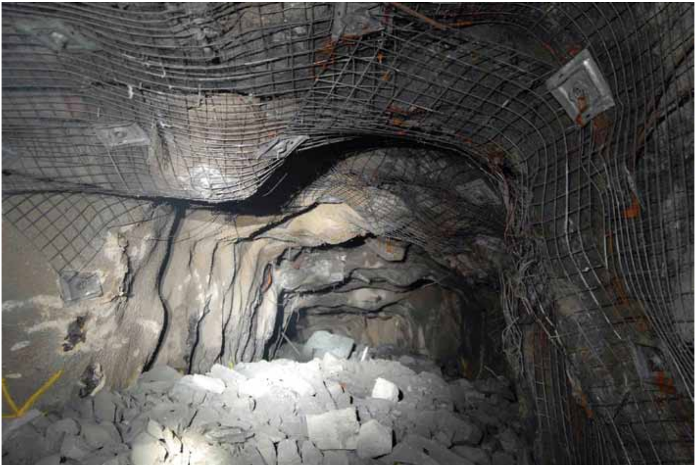
Fig. 4: FRS with mesh over the top in a high-stress Western Australia mine
