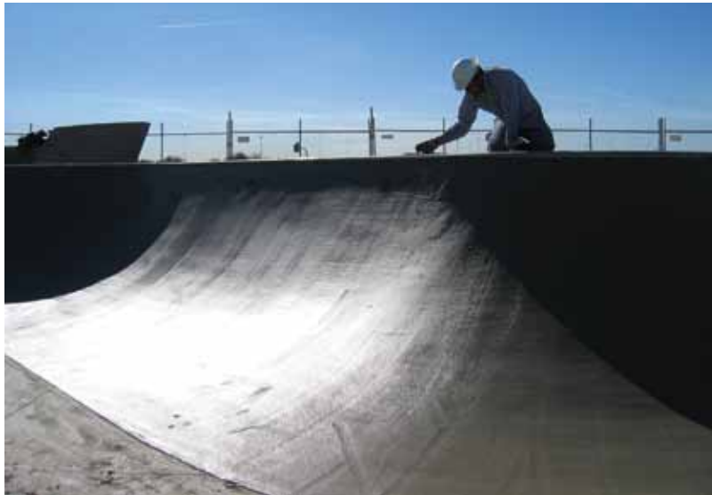
This Peoria, AZ, municipal skatepark had to have an ultra-smooth finish for the safety and experience of the user
