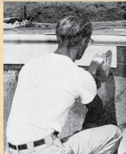
Tile and coping set around pool's edge by skilled craftsmen serve to make maintenance easier as well as add decorative touch
