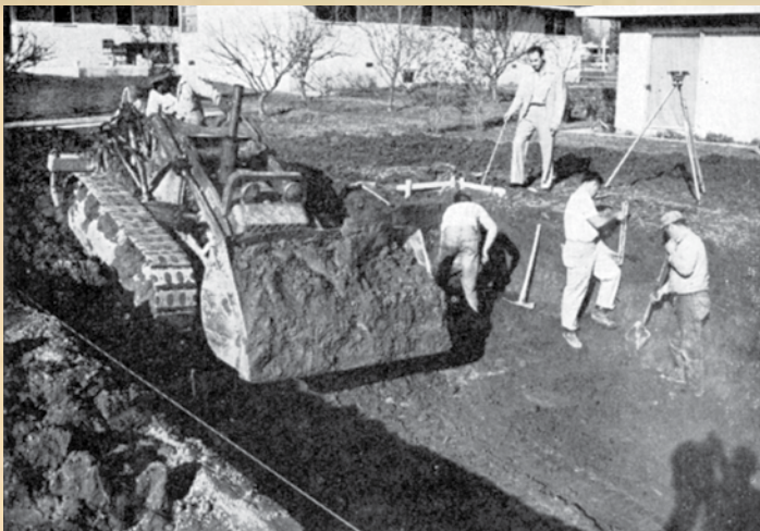
Excavation being done here with a Hough Payloader; which ramps out of shallow end of pool. Proper setting of forms and excavation are two crucial operations
