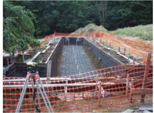
A residential pool prior to the shotcrete process. Pipes are capped and pressurized to ensure the system has no leaks
