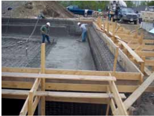
This is a straight, solid formwork and steel application of concrete being placed and is one of the items on the check list for proper placement
