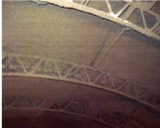
Lattice girder tunnel supports within the layers of fiber-reinforced shotcrete (initial layer)
