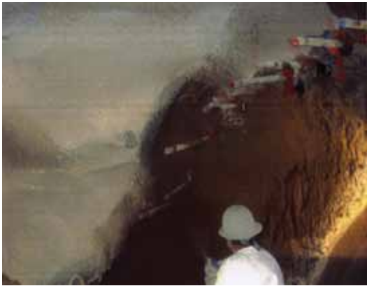
Shotcrete being applied near portal area. Spiling installed and shot in prior to the demolition of the adjacent panel
