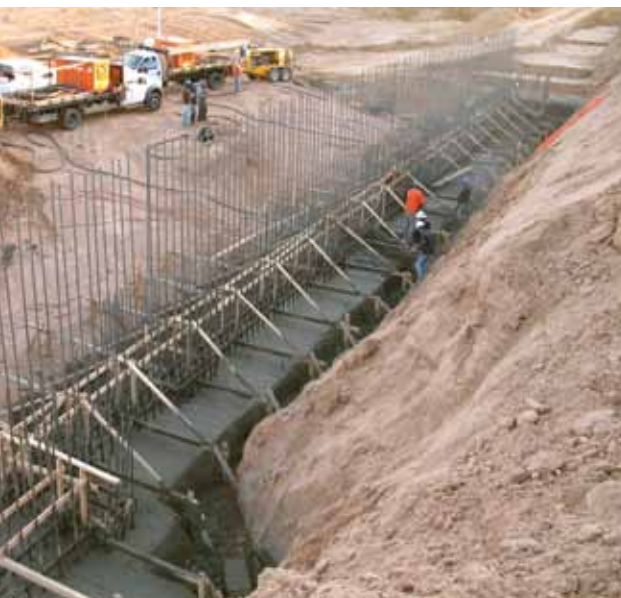
Shotcrete being placed for one of the faux bridge retaining walls. A total of 180 yd 3 (138 m 3 ) were placed in one shift for each of these massive footings
