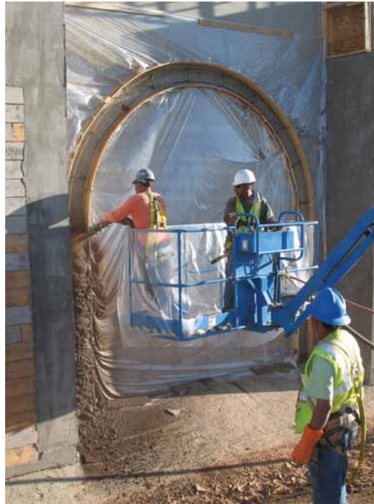
Placing colored shotcrete for the arched sills on the bridge walls. Note the board-formed sections within the water columns
