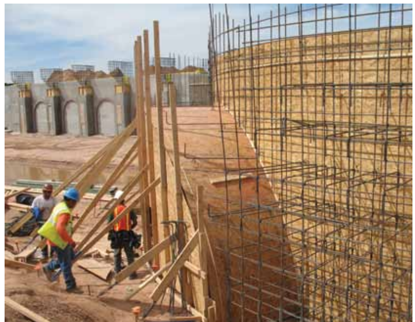
The two sign walls presented numerous forming challenges. This is a 6 ft (1.8 m) thick wall with an arched opening within a curved section
