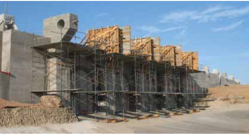
Access for forming the water column crowns was from scaffolding 20 ft (6 m) off the ground on both sides of the wall
