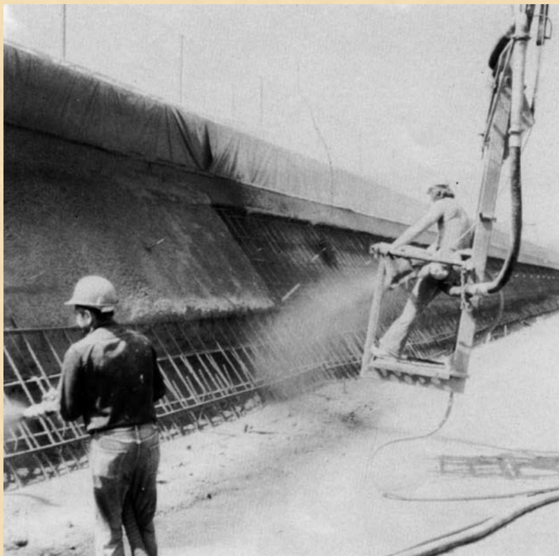
Shotcrete is often placed from a boom bucket as well as from grade level
