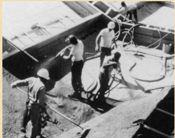
Because of the high compaction density achieved by air placement, finishing operations can start immediately
