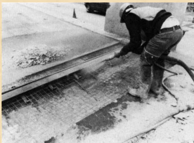
Shotcrete expansion dam became loose, had to be rewelded
