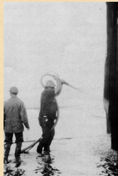
Shotcrete being applied over existing wood piling that had considerable erosion damage. By use of mesh-reinforced shotcrete, the pier was salvaged and is back in use
