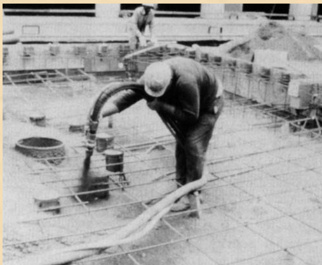
Water-jetting equipment from a fountain is being encased in air-placed concrete. The nozzleman is directing the stream around this equipment to ensure proper imbedment
