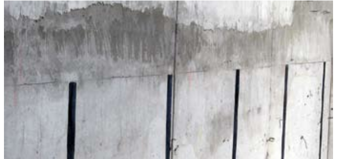
The overspray makes the wall appear unfinished and in need of repair. The vertical strips are metal imbeds used for durability. This is a bin for recycled material
