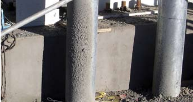
Thin overspray on a pipe. Don't think that because it is thin that it will be easier to remove. Sometimes the thinner layers are harder to clean
