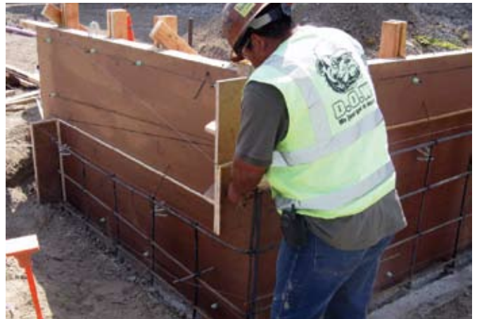
Small concrete walls and planters are installed using a single form. Chamfer is installed for elevation change. Piano wire is set up at the face of the wall and shot using the wet-mix shotcrete process. It's simple and quick
