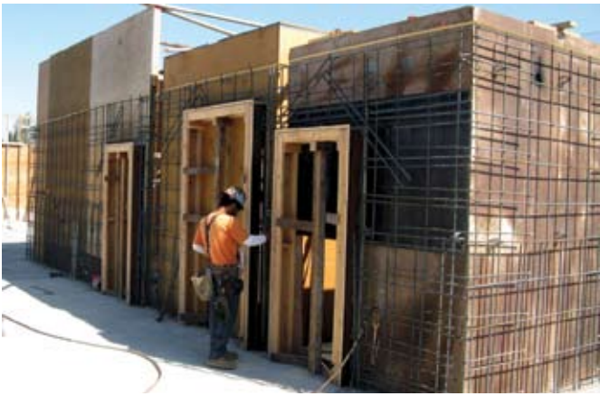
Elevator forms with door openings ready for construction using the shotcrete process
