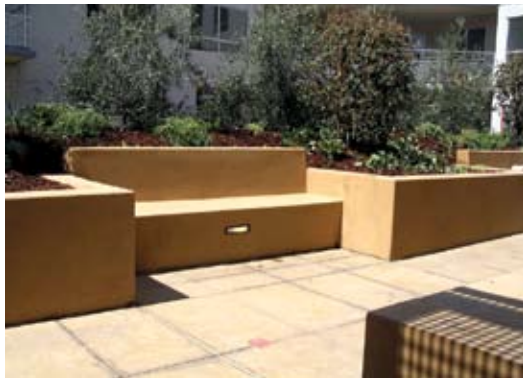
Completed shotcrete bench project with colored shotcrete installed with a smooth trowel finish
