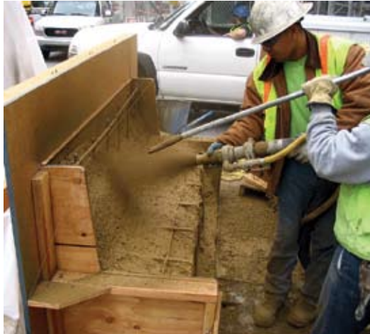
Shooting concrete benches with color for a landscaped courtyard on a podium deck in San Francisco, CA. All forming was built free-standing and held in place with sand bags so no nails would penetrate the podium deck waterproofing
