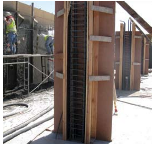
Note that even the pilaster forms are installed for construction with the shotcrete process with a simple form and chamfer used to establish line and grade
