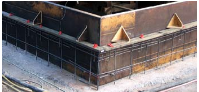
This is a simple residential foundation. Back form, mud sill, and bolts are installed. Shotcrete will be installed on the face of the mud sill. When complete, it will be equivalent to a concrete foundation with sill and bolts installed, saving time and money
