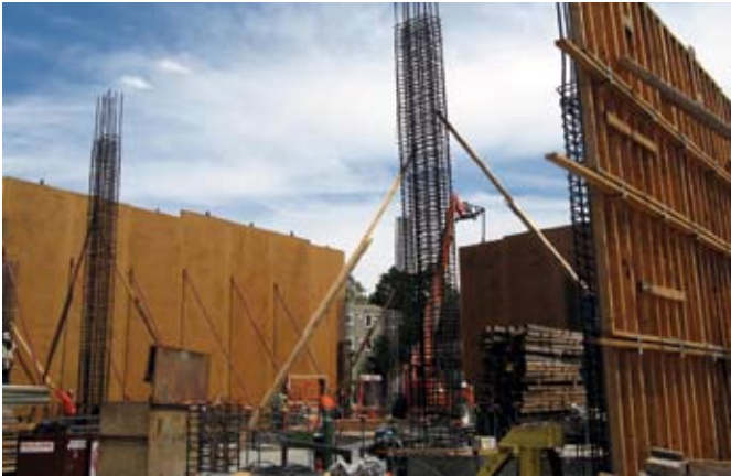
This photo illustrates tall wall forming. Forms are prebuilt in a fabrication yard off site and then shipped and set by crane using pipe shore bracing
