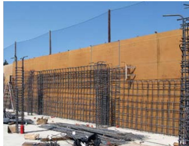
This photo illustrates how elevation changes can be installed in the wall. Wall forms are installed past full height, and a chamfer reveal is installed at the top of the wall
