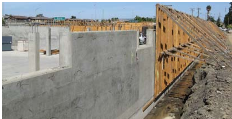
This photo shows how simply a back form for a wall can be installed; note how clean the stripped face of the installed shotcrete wall is
