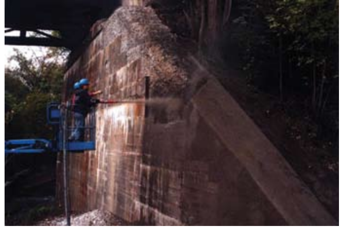
Dry-shotcrete work to a bridge abutment on the Western Maryland Scenic Rail Road in Cumberland, MD
