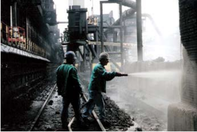
Dry-shotcrete process to repair a quench tower at the United States Steel, Clairton Works, Clairton, PA, in 2006
