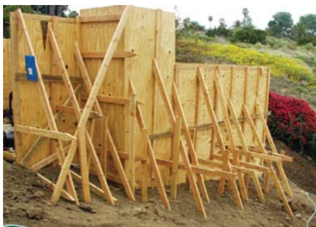
Fig. 3: The most difficult and complex forming is required when a swimming pool is built either partially or completely out of grade
