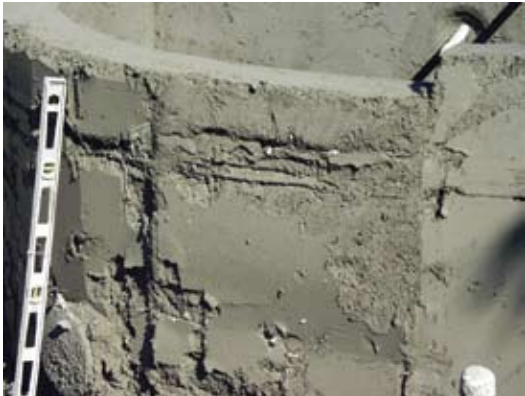
Fig. 8: Delamination occurred when forms were stripped. The surface against the form contained sand lenses and trapped overspray and rebound
