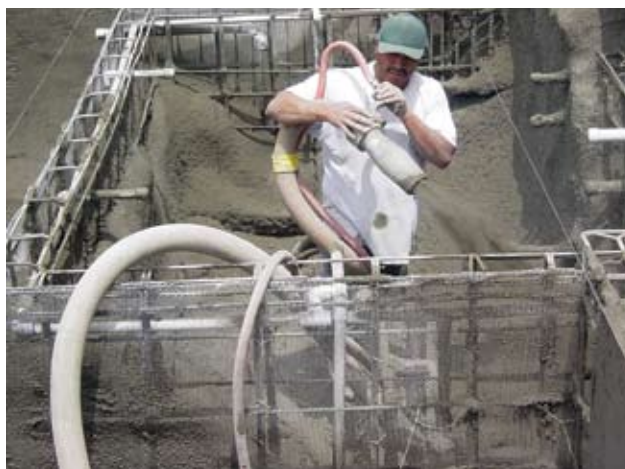
Fig. 4: Another questionable practice: an expanded metal lath is tied directly to the reinforcement and left in place between the inner and outer layer of shotcrete
