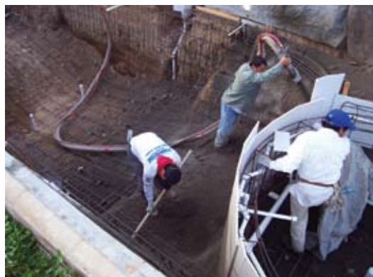
Fig. 6: Drywall form often placed on the outside of the reinforcement and the wall shot from the inside. Only tie wire on the outer face is holding the drywall in place
