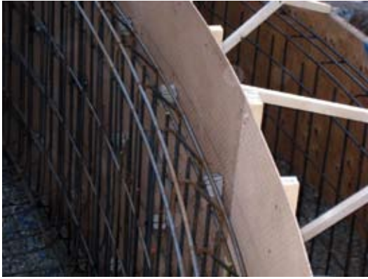
Fig. 7: Example of secure dam wall forming braced to resist vibration and the impact force of the shotcrete. Reinforcement tied to forms with dobies to resist vibration and provide proper coverage
