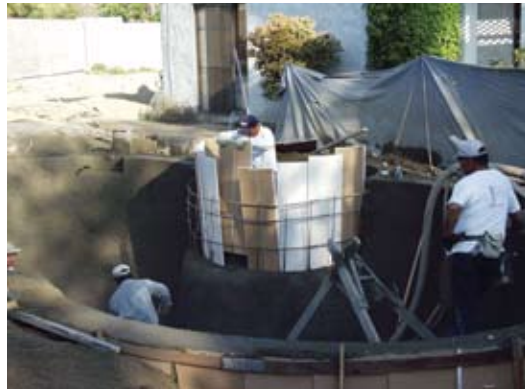
Fig. 5: Unacceptable practice: drywall form held directly against reinforcement by crew member without dobies or spacers to establish the cover over the reinforcement
