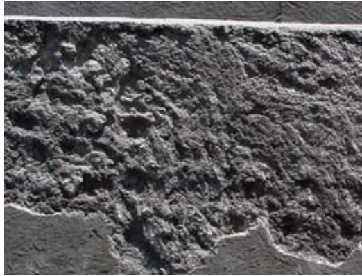
Fig. 9: After the forms are stripped, this becomes the receiving surface for shotcrete on the alternate side. Results in questionable bond and reinforcing bar encapsulation
