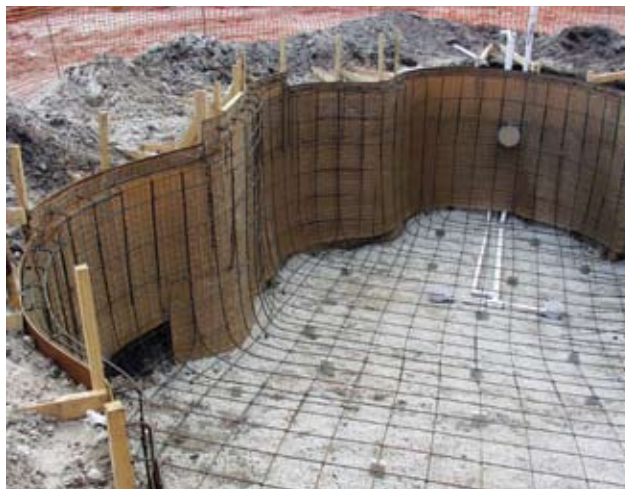
Fig. 2: In Florida and several areas of the northeastern U.S., the perimeter of swimming pools is often over-excavated then usually formed using steel-tex, a paperback wire mesh
