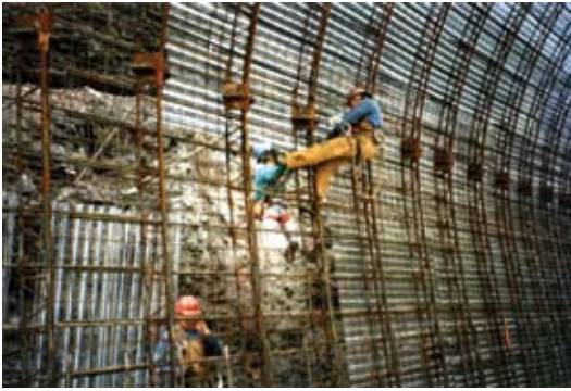
Figure 3: Men working on wire tying Stay-form to lattice girders and reinforcing bars
