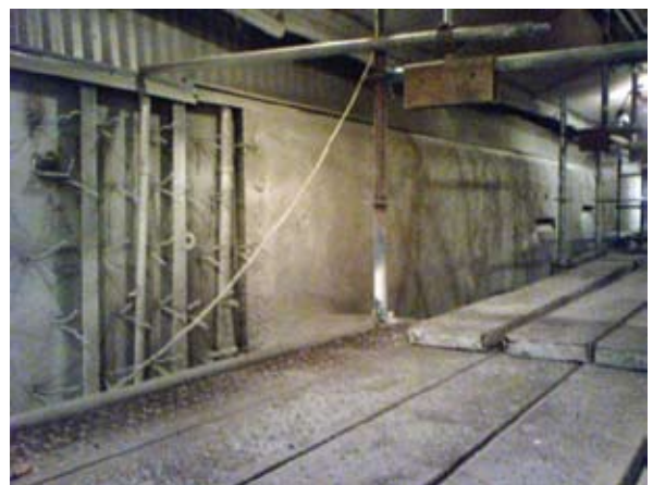
The ungunned area to the left shows the V-Type refractory anchors with monolithically gunned refractory
