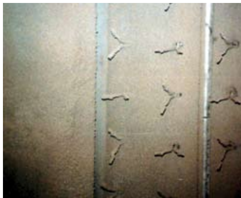
Ash hopper sidewall (left) with the refractory gunned to full 9 in. (229 mm) depth and V-anchors (right)
