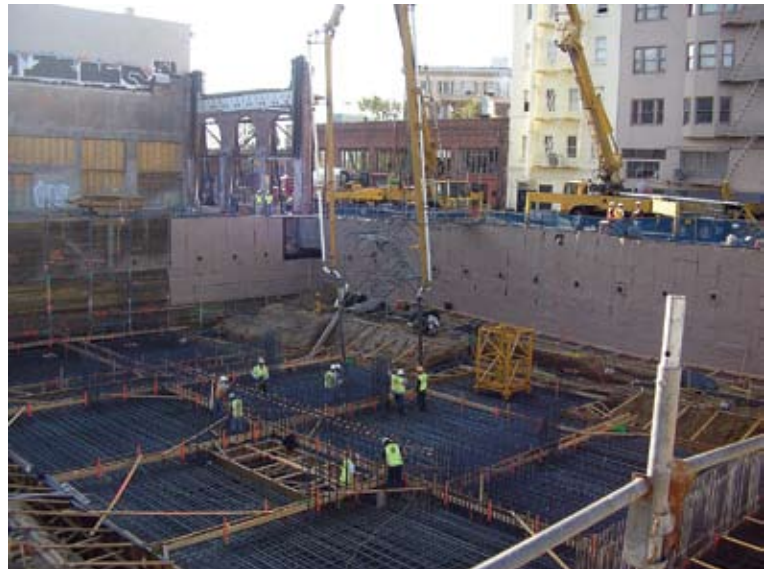
Fig. 2: Example of a clean site from the top of the southeast stair tower (55 Page Street in San Francisco, CA)
