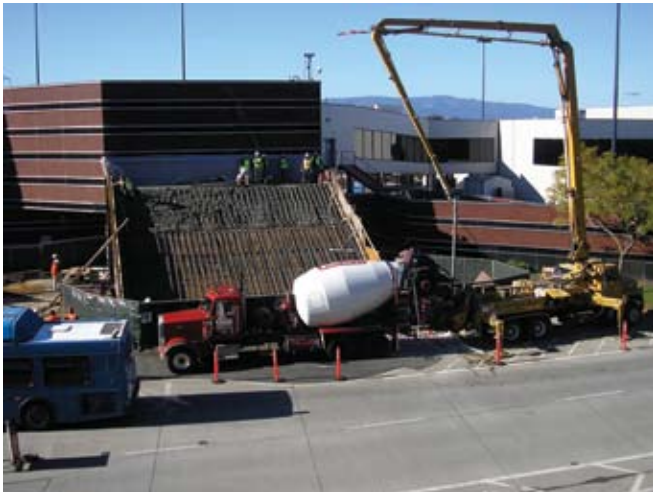
Fig. 4: Example of good work plan in action (San Jose Airport, Terminal A)
