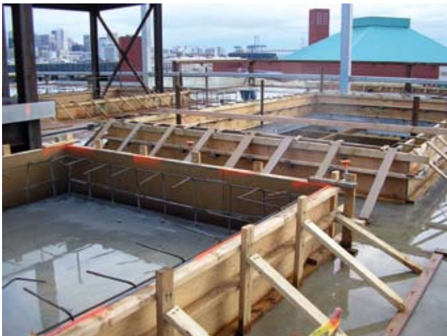
Fig. 5: Example of a clean job site with multiple forms at roof—good job planning and execution of work (Mission Bay Life Science Building, San Francisco, CA)
