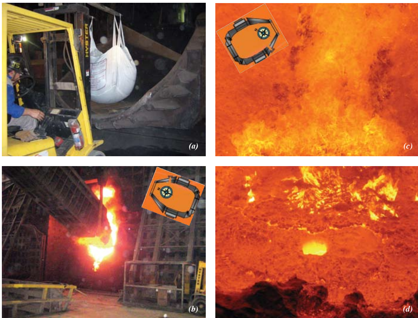
Fig. 3: BOF hot-repair procedure: (a) loading R2U MgO-C castable on scrap crane; (b) castable is applied at the impact pad; (c) castable flows to the tap pad; and (d) castable is set and BOF is ready to resume operation. Illustrations inset in (b) and (c) indicate ladle orientation at those points in the process
