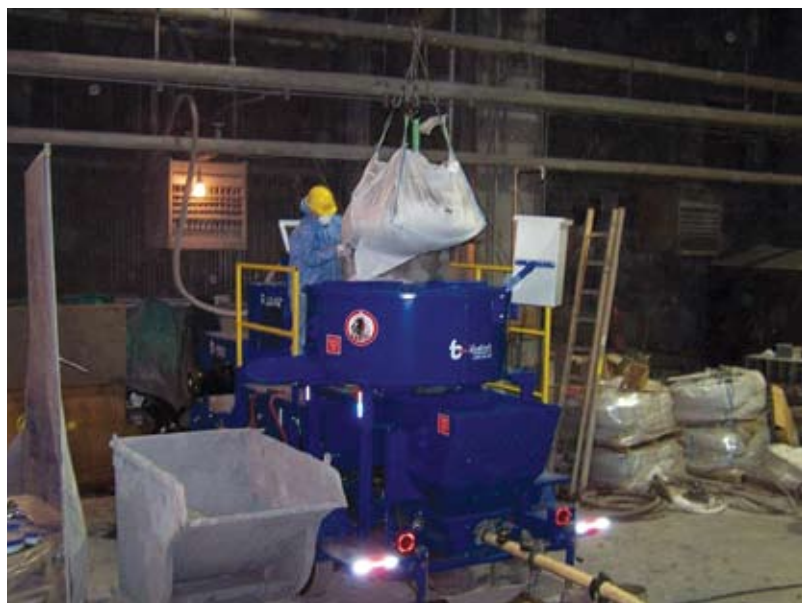
2200 lb (998 kg) bulk bags are loaded into a mixer and ultra-high-pressure pump for wet shotcrete process
