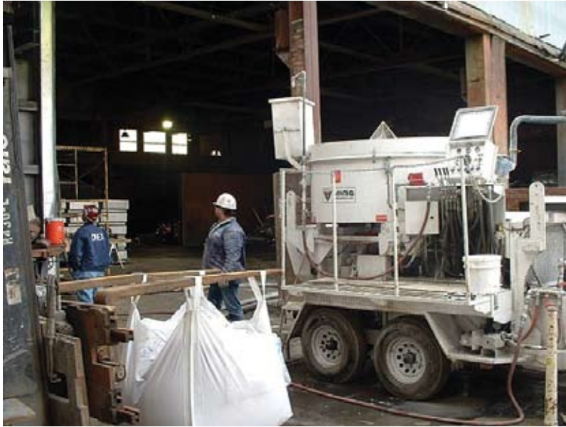
A typical setup lining a cement kiln with wet shotcrete refractory material
