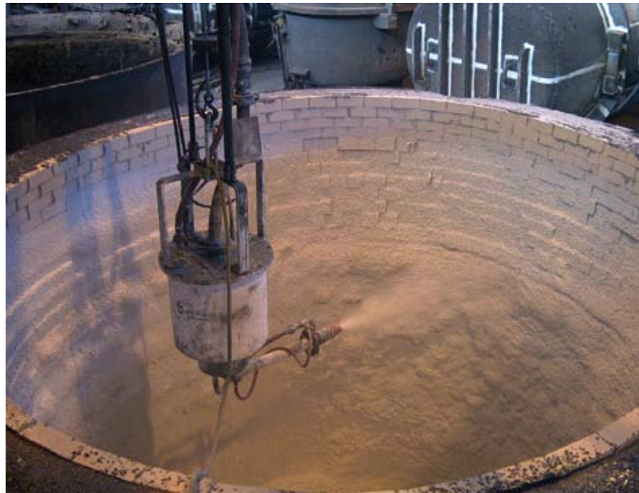
Robotics are used for spraying ladles with wet shotcrete at North American Refractories’ ladle maintenance facility in Gary, IN
