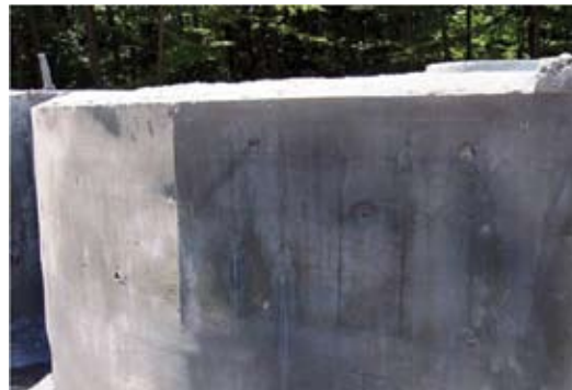
Back of vanishing edge wall that receives tile. Notice the wood grain mirroring on the concrete (high-velocity, good density)
