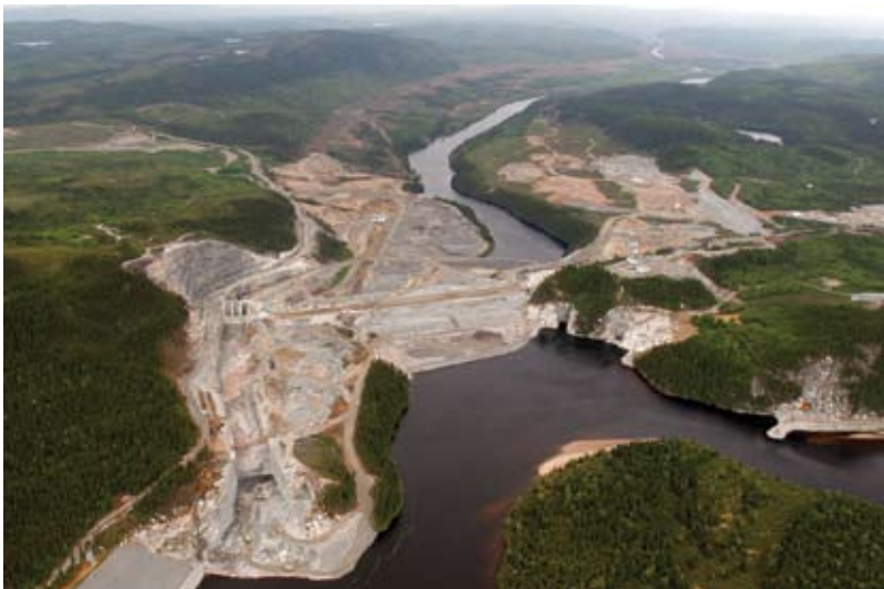
Fig. 5: General view of the project on the Péribonka River, June 2007 (Photo courtesy of Hydro-Québec)
