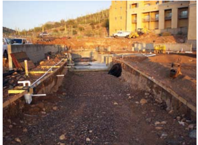
Partial excavation of the last section left for access to island. Here is an example where the joint detail was formed incorrectly, where the integrity of shooting the subsequent lap beneath the floor cannot easily be validated
