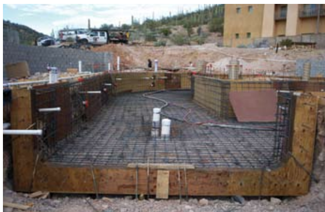
A section ready for shotcrete with form joint in place. Peg board installed behind steel to save shotcrete material from filling voids in poorly consolidated soil in excavated walls, later backfilled with pea gravel
