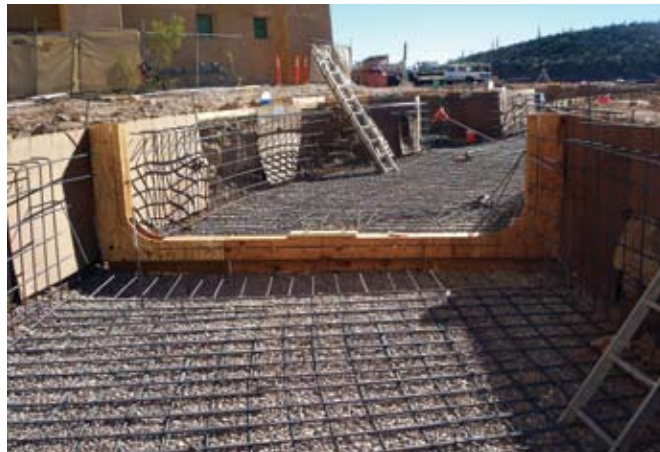
Forms are constructed in sections for ease of removal and set prior to completing steel placement. Installing waterstop and 1/2 in. (13 mm) stainless steel rods will finish the form preparation. This photo shows a side view of the shotcrete placement
