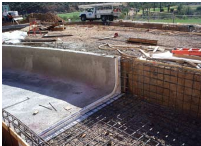
A finished shotcrete joint section with 5/8 in. (16 mm) foam separation installed, ready for next shoot
