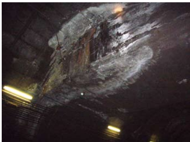
Typical delaminations on Red Line tunnel at B Street
