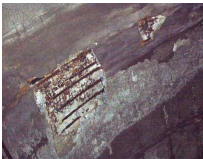
Delamination in arch of tunnel lining
