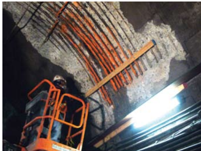
Close-up of delaminated area after removal of the delaminations
