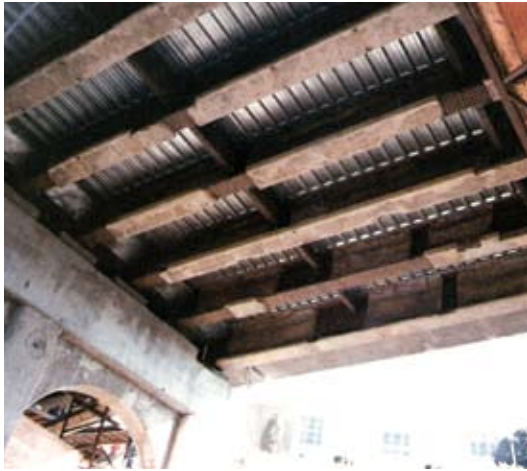
One of the spans after the damaged shotcrete was removed and the anchors and mesh were installed
