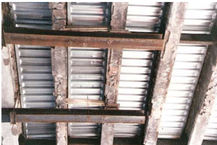
Damaged beams on one of the spans
