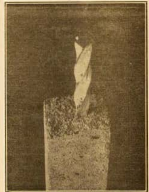
FIG. 5.—SHOWING SPURS OF RUST ON METAL OTHERWISE PROTECTED BY MORTAR
