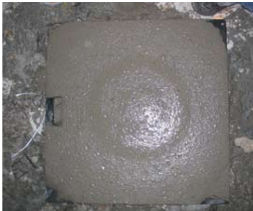
Fig. 3: Slump-spread of shotcrete mixture of September 4
