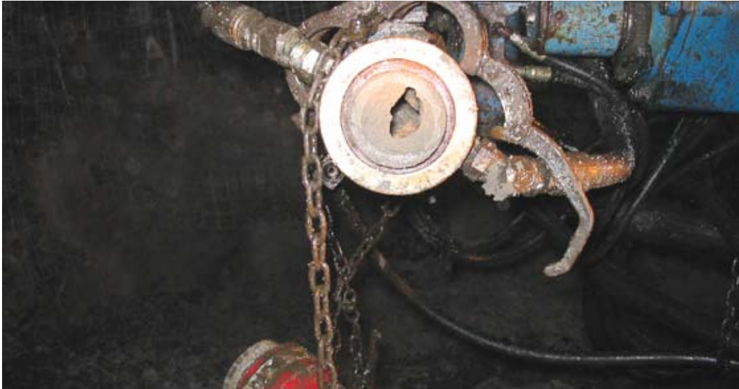
Fig. 10: Accumulation of shotcrete in the nozzle
