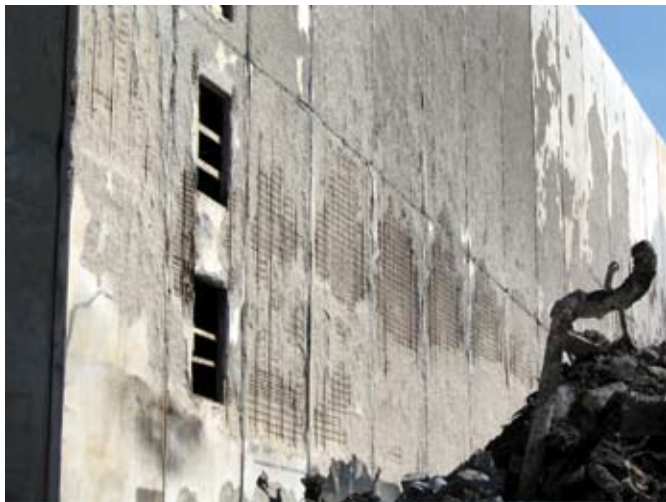
Overall view of portion of the garage where damage was severe and many panels were replaced. Only limited testing was conducted on these panels
