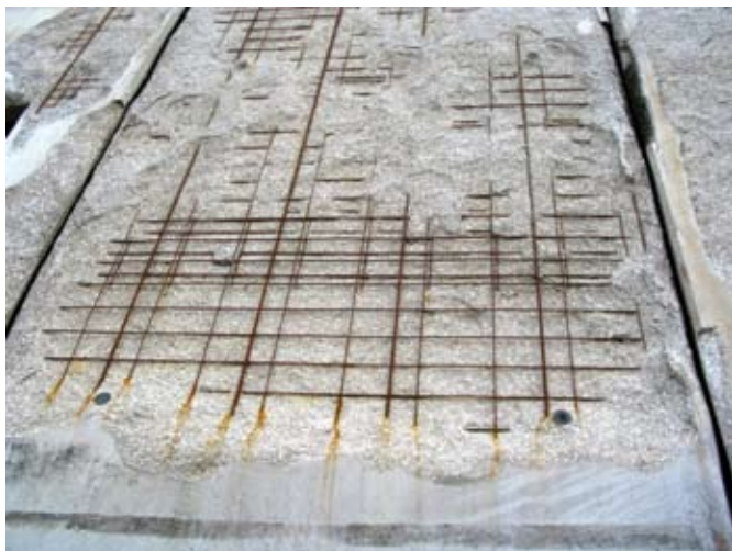
Common degree of damage suffered at the precast panel exterior face due to fire. Spall depths of up to 2-1/2 in. (6 cm) exposing steel were not uncommon
