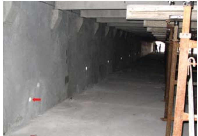
Overall view of typical interior panel faces. Core holes are visible. The inside faces of the panels were generally unaffected by the fire and provided an excellent surface to send and receive impulse signals
