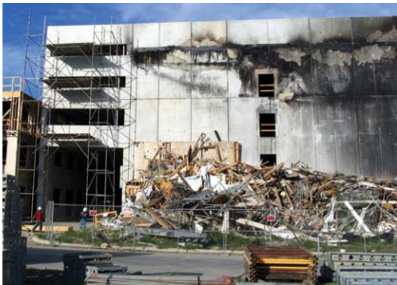
Overall view of garage wall at entrance. Debris is still in place at the time of the site visit, preventing visual inspection of exterior surfaces of lower panels. However, NDT proceeded as planned from the interior surfaces
