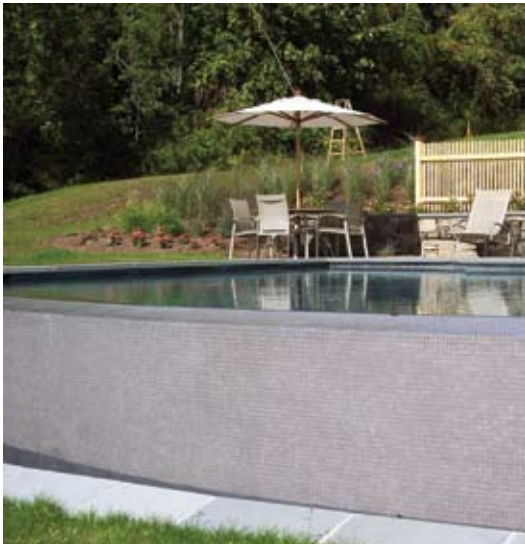
A view of the edge wall shows the finish materials in place. Tolerance for the edge wall upon completion of the tile is \pm 1/32 in. (1.5 mm). The flow of water over the edge is minimal if executed properly
