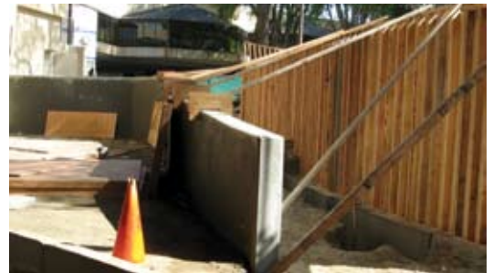
Simple wall forming was used at the radius wall on the right. All the wall slopes and gutters were constructed with 4000 psi (25 MPa) shotcrete
