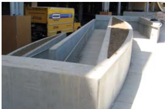
Areas of the walls and ramps all constructed using the shotcrete process (this work was completed in one day). All the walls have a trowel finish with tooled chamfer at top. The only sacking done on the project is on the form side. Smooth form plywood was used so sacking was kept to a minimum, saving another week on the schedule
