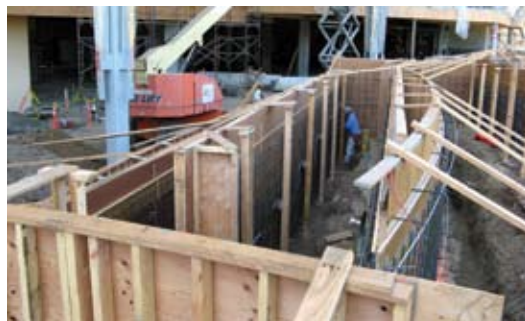
A fast single-forming system. Forming detail was used at the top of wall along with a chamfer used for the screed point. Note the 2 x 4 in. (51 x 102 mm) timber at the face of the wall for placement of lights. Fiberglass rods were used for the top of the wall elevation to produce the radius at the top of wall. This project had a series of walls and ramps, and as soon as one set of walls was completed, the forms went up for another
