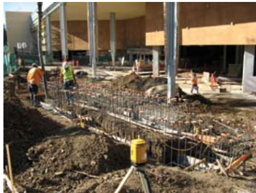
The footing of one of the areas being poured along with the demolition of the parking area (approximately 25 days to complete the project)
