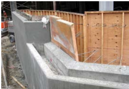
A completed section of the water feature. Areas shown were completed monolithically using both pump and vibrate and shooting techniques
