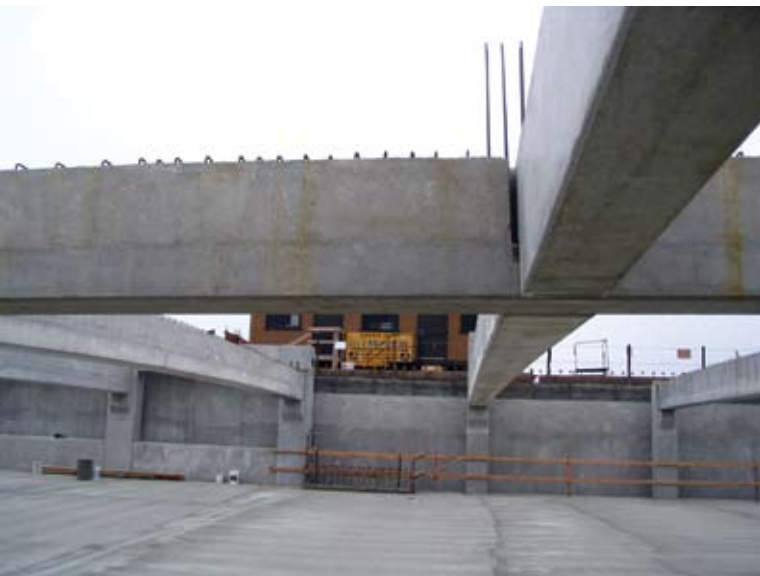
Precast beams, shearwalls, and retaining walls complete and ready for deck forming and reinforcing
