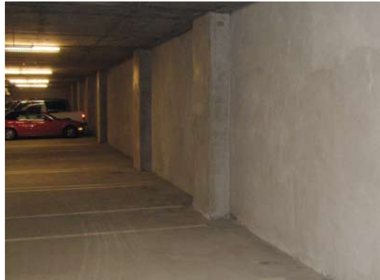
View of the completed walls and pilasters (constructed using shotcrete as the placement technique)
