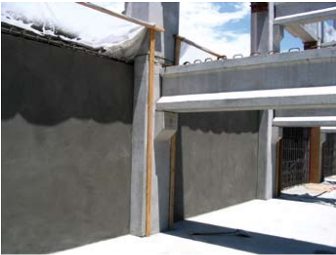
Completed 4000 psi (28 MPa) sand float finish walls (installed by the shotcrete process)
