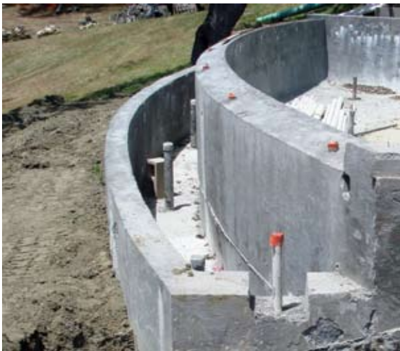
On vanishing edge pools, the weir wall and often the outer basin wall must be formed for shotcrete application. Forms are usually erected on the outside of the wall
