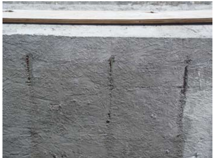
The dobies slipped out during shotcrete application, allowing the reinforcement and formwork to come together, leaving essentially no cover over the reinforcement
