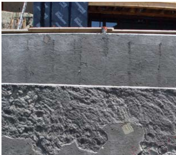
When the forms were stripped, the outer surface of the basin wall delaminated, leaving substandard cover over the reinforcement. Note the exposed reinforcement in the weir wall in the background
