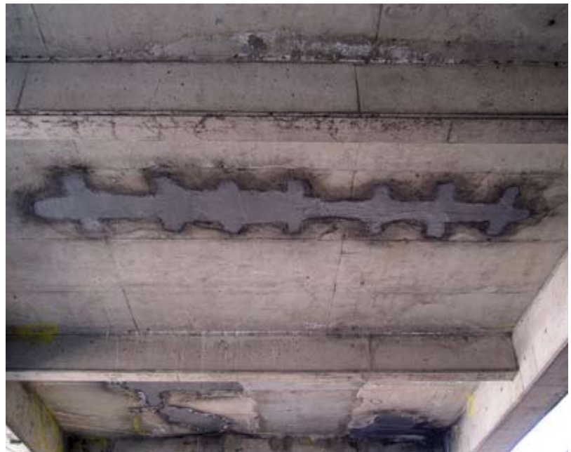
The same area shown in the first photo, after repair. The pattern of the shotcrete in the foreground is where additional concrete was removed to get sufficient development length for the new reinforcing steel that was added
