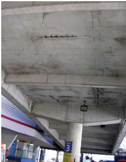
One of the repair areas prior to intervention. Note the extensive spalling
