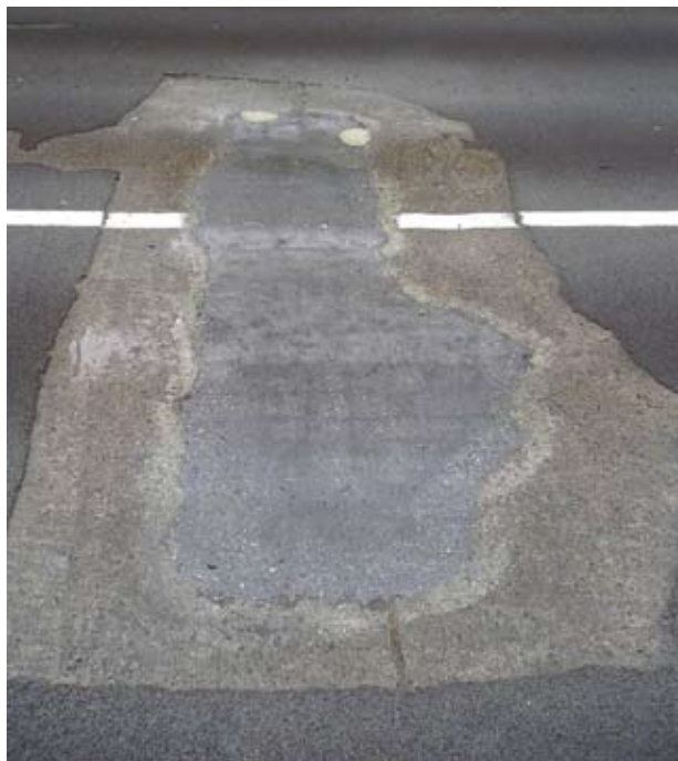
The top formed side of a typical through-patch. The light spots at the ends are where small voids were repaired
