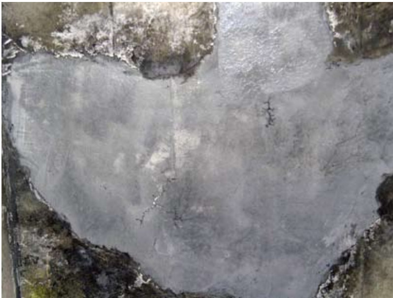
A typical patch from the bottom. Some minor restrained shrinkage cracking was noted in both the shotcrete and the cast-in-place patches
