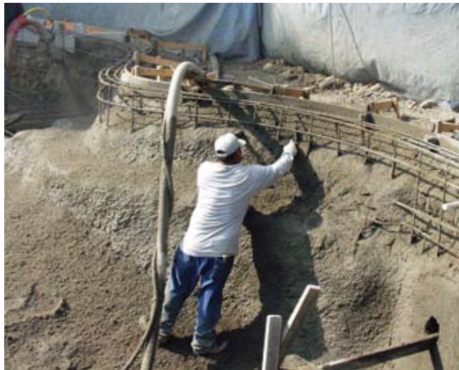
Joints standing for over 30 minutes must be cut to a 45-degree angle then cleaned and wetted before placing additional shotcrete and safety practices must be followed
