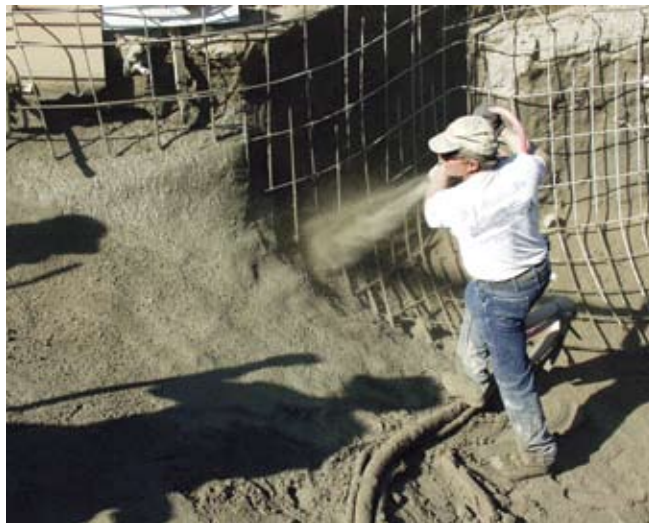
Shoot the cove and the floor at the base of the wall before the wall is shot to eliminate rebound, overspray, and trimmings from becoming trapped at this critical location and practice proper safety procedures
