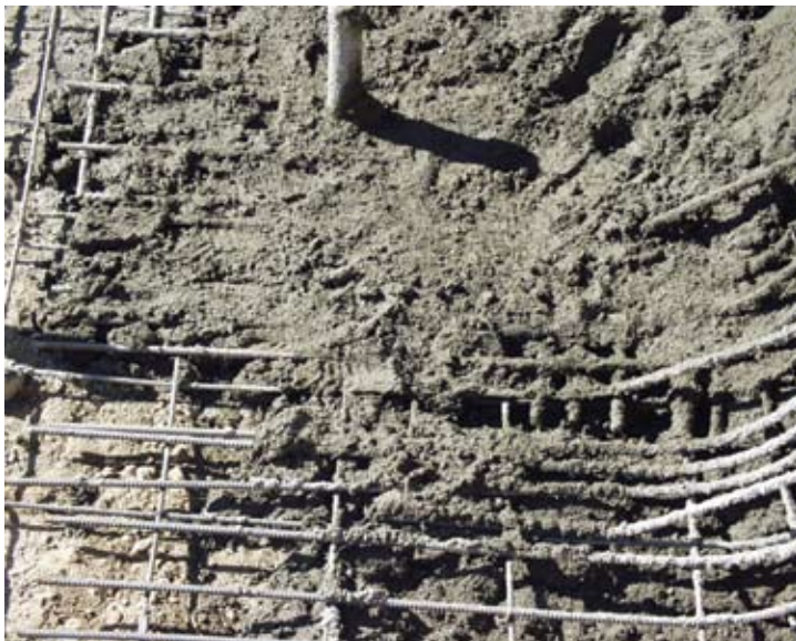
This trimmed material sat in a pile at the base of the wall for over 90 minutes. Remember, concrete consolidation and reinforcement encapsulation are critical elements of structural concrete placement
