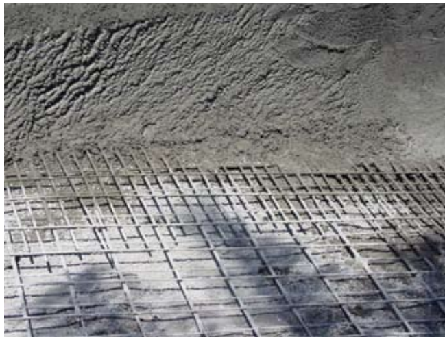
Here's a typical joint that stood for over 30 minutes—notice the overspray and rebound. No cleaning and wetting took place before placing new material
