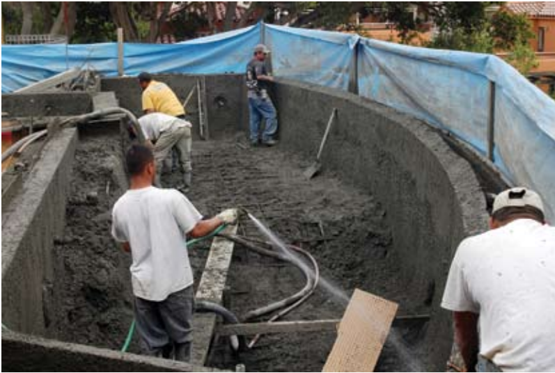
In addition to poor placement practices, proper safety practices are not being followed here
