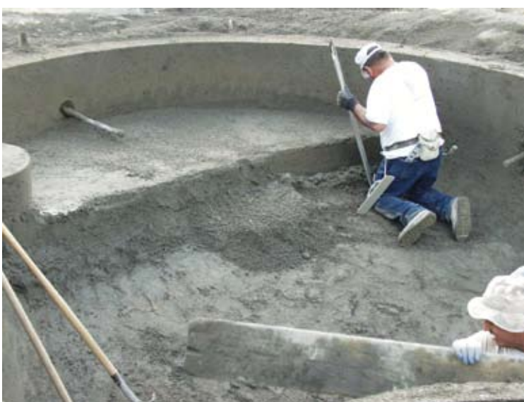
The origin of the problem seems obvious: it has to do with the use of gunite rebound in shaping steps and benches. This material has no structural value in a pool shell: It should be gathered up and discarded—no exceptions!
