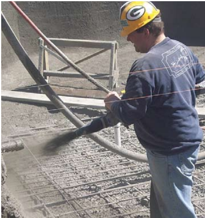
Shooting for exact tolerances on walls and edges creates ease of movement for water in transit. Shooting in tight tolerances also reduces preparation for the installation of the finish material
