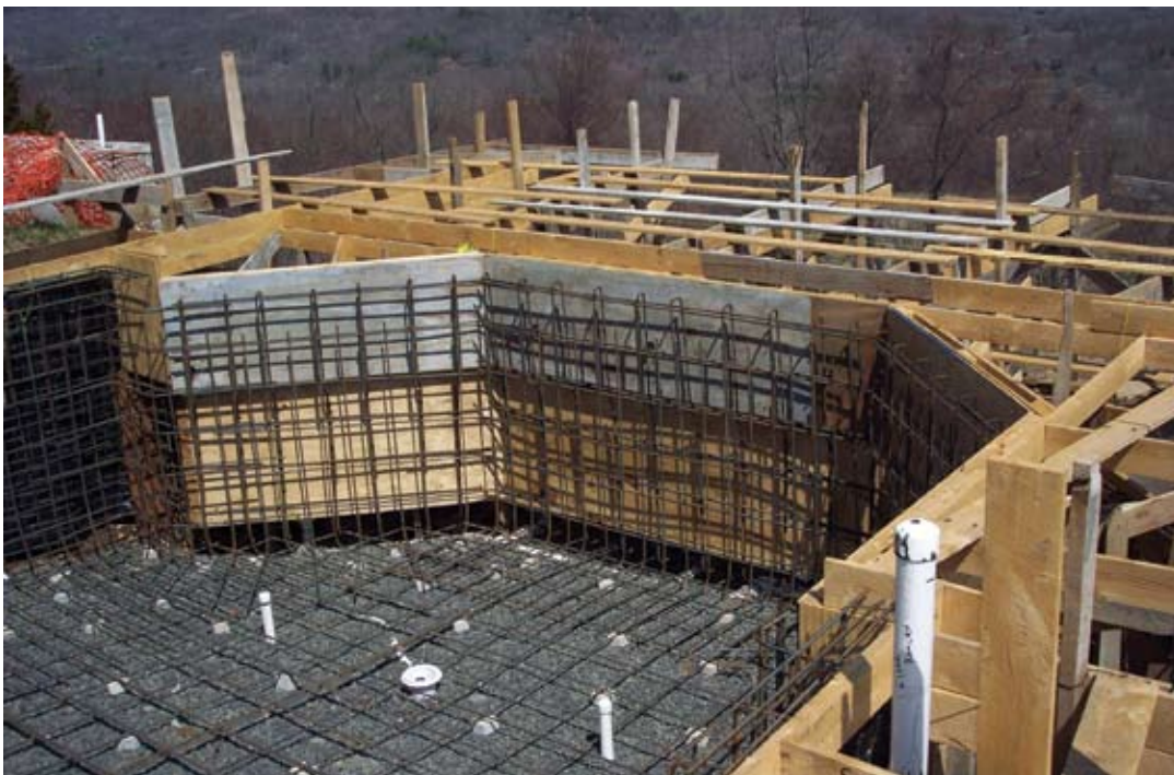
This picture shows a double cage steel and rough sawn lumber for out of ground construction
