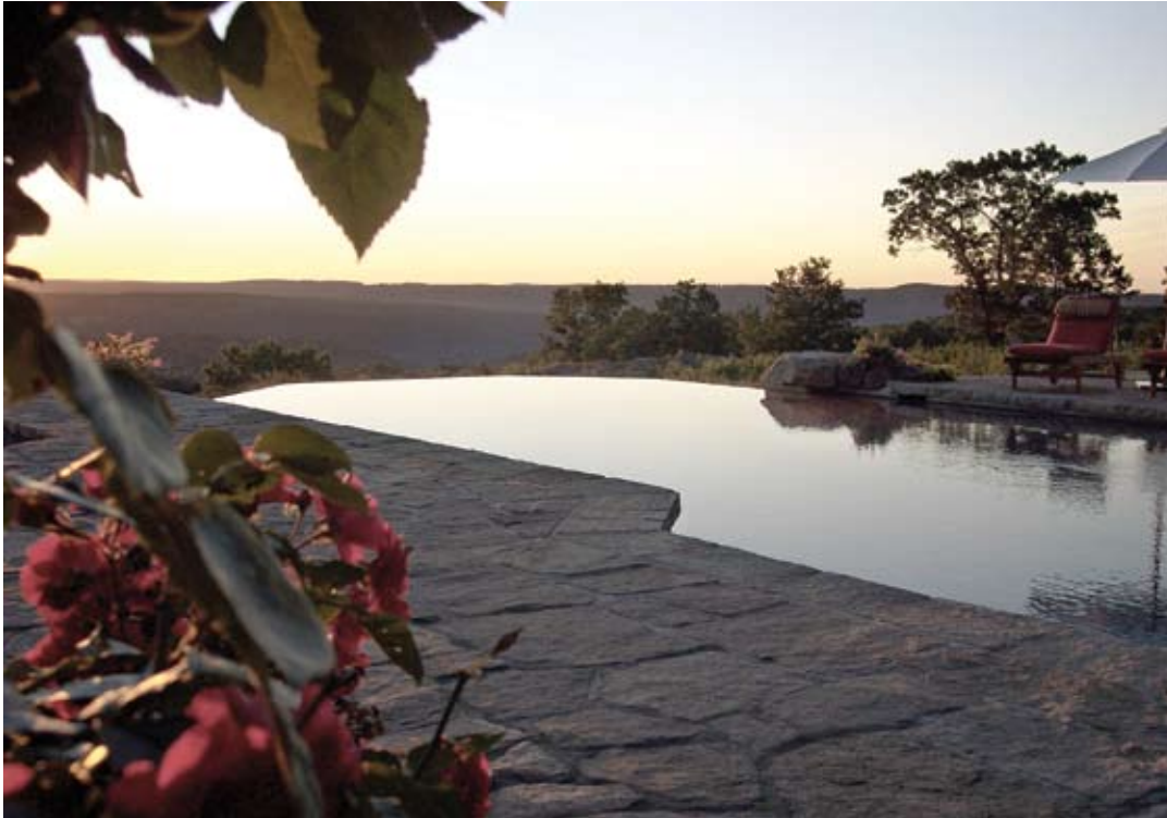
The precise tolerances of the shotcrete create the perfect edge. The execution is critical and will show any flaws in the finished product
