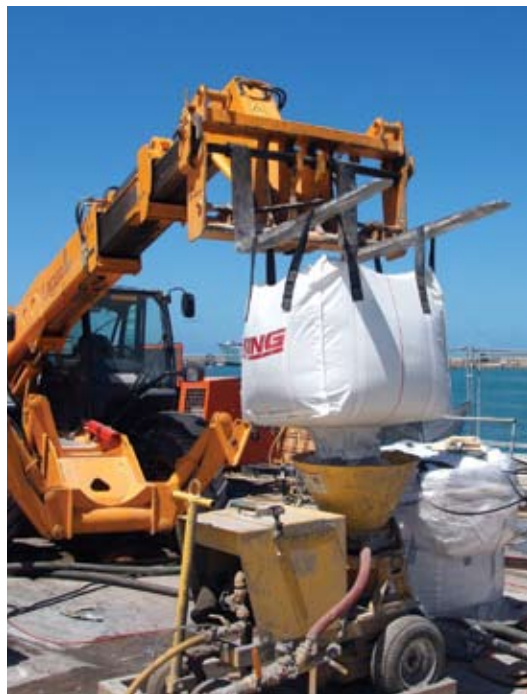
Fig. 4: Shotcrete machine and bulk bags containing the preblended materials were positioned on the top of the slab while shotcrete was applied underneath
