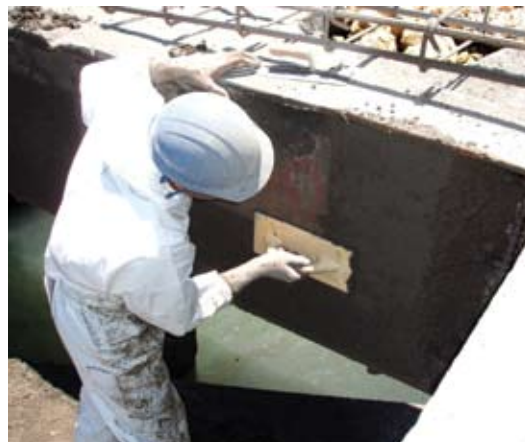
Fig. 5: Finishing had to be completed quickly because of the affect that hot temperatures had on the plastic properties of the shotcrete mixture
