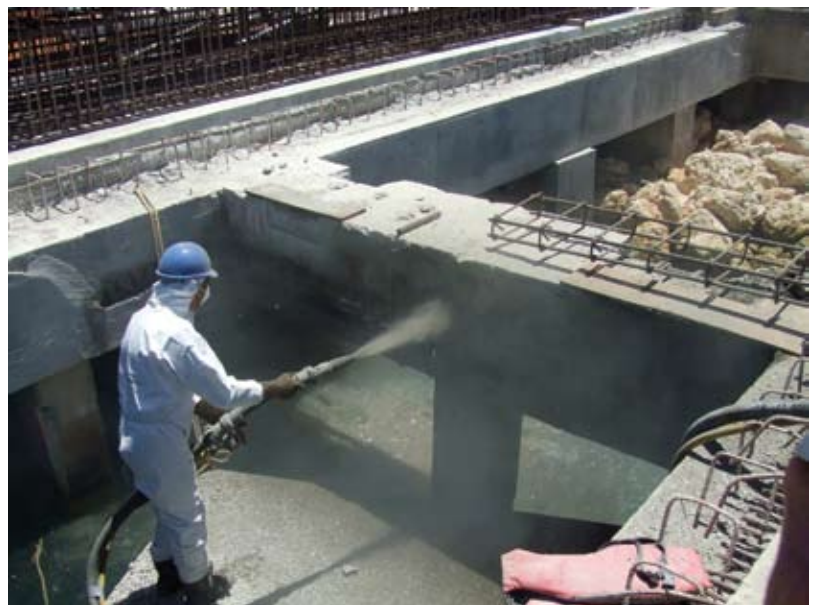
Fig. 3: The shotcrete hoses ran from the shotcrete machine, which was stored with the prepackaged materials, on the top of the slab to the nozzelman who was positioned below the slab, just above the surface of the water
