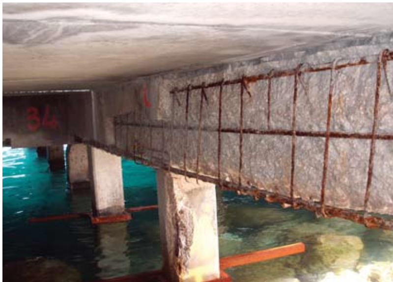
Fig. 1: Severely deteriorated concrete beams (after concrete removal)
